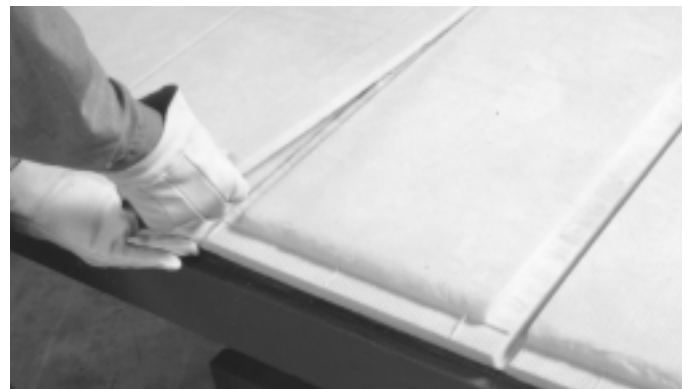
Fig. 2-11. Remove groove scrap. Confirm dimensions. The board is now ready for assembly and closure of a straight duct module, or for fabrication of a fitting.
