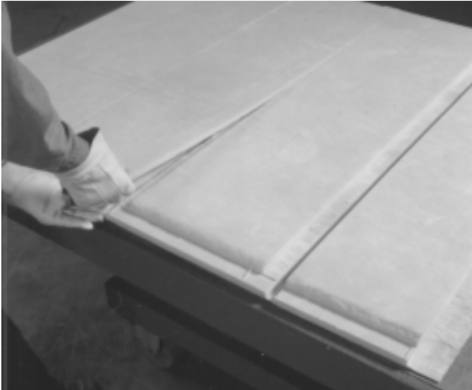
1. Cut shiplaps and corner grooves with hand tools or by machine as shown on pages 2-12 through 2-15. Remove groove scrap. Lifting board as shown will make it easier to remove shiplap groove scrap.
