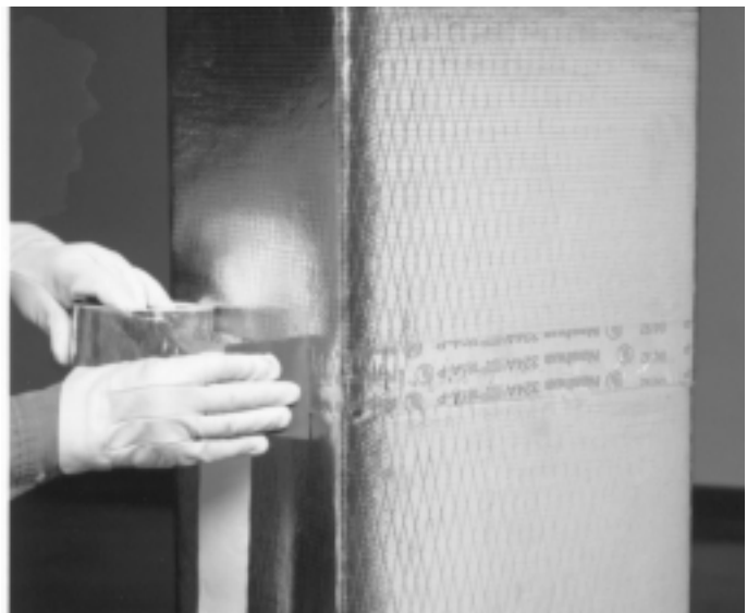
4. Complete closure of circumferential joint with UL 181A listed closure. (Pressure-sensitive tape shown above.) Duct board surface must be clean and dry.
