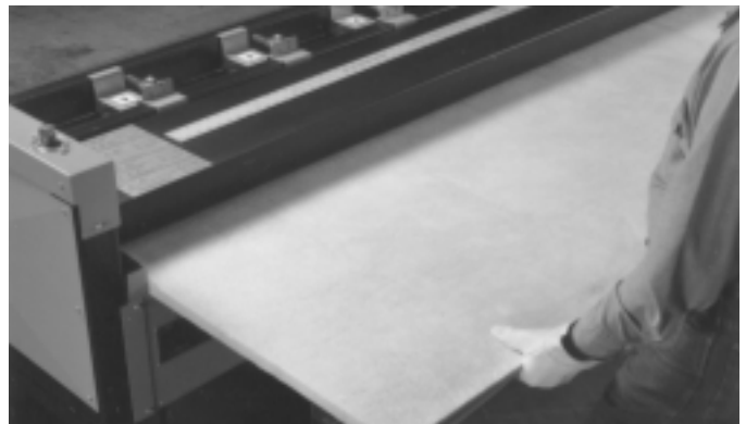
Fig. 2-10. Feed duct board into machine, female shiplap edge first, left hand edge firmly against guide, parallel to rollers. Turn on machine and guide board as friction rollers pick it up and pull it through the cutting tools.
