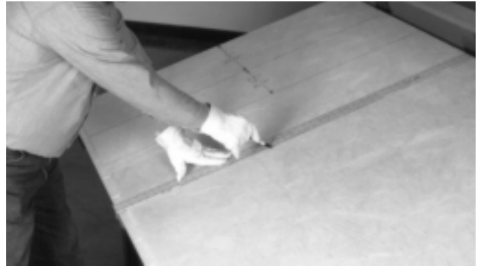
3. From there, measure 12" (305mm), same as first inside duct dimension, + add-on allowance of 1\frac{3}{4}" (44mm), total 13\frac{3}{4}" (349mm). Draw third corner groove centerline.
