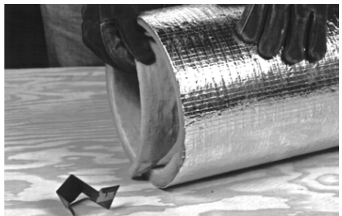
Fig. 7-2C. Using shiplap cutter to make female shiplap. Cutter is positioned to cut into inside of duct wall.
