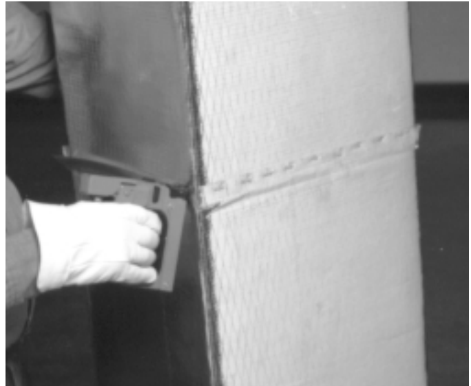
3. Staple flaps on all four sides with 2" (50mm) (approx.) on centers. Use outward clinching staples, galvanized steel, 1/2" (13mm) long, crown width 0.400" (10mm) (min.), flat wire 0.040" x 0.020" (1.0 x 0.5 mm) (min.).
