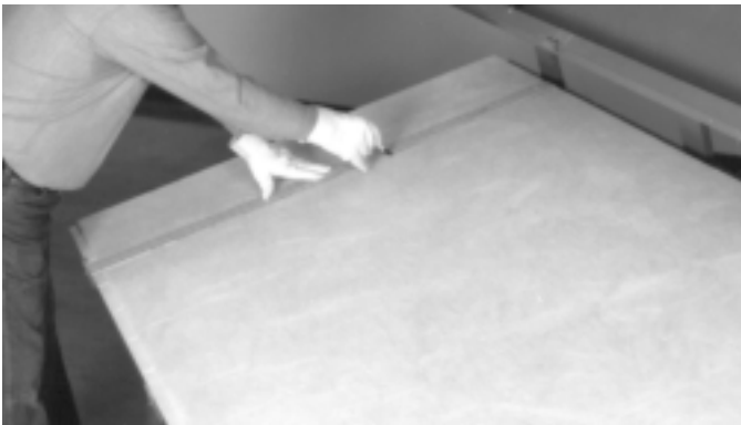
1. With factory female shiplap toward you, from left edge of board measure 12" (305mm) (first inside duct dimension) + add-on allowance of 1\frac{3}{4}" (44mm), total 13\frac{3}{4}" (349mm). Draw first corner groove centerline.
