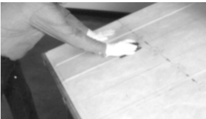
8. Rotate modified shiplap tool end for end (or use next sequentially numbered tool) and cut along second corner break centerline so right side of panel #2 is cut straight and shiplap is on left side of panel #3. Lift board slightly and remove groove scrap.
