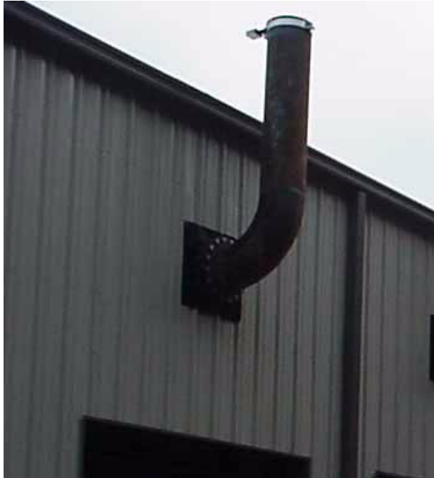
Figure 6–9. A Simple Exhaust System Fitted With a Rain Cap to Prevent Rain From Entering the Exhaust.
