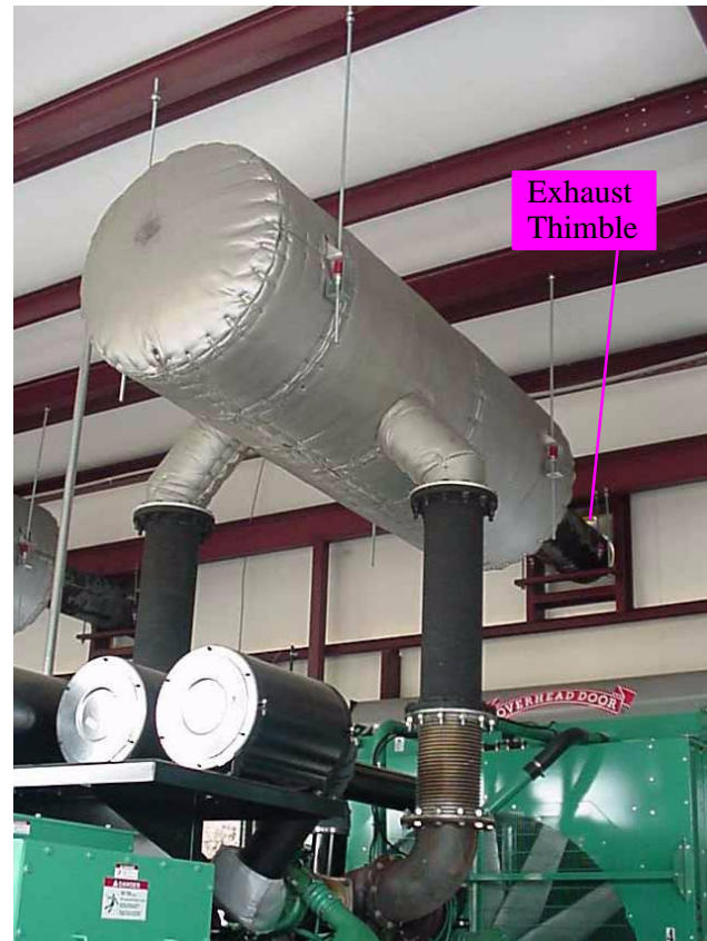
Figure 6–7: Generator Set Exhaust System Features. Dual Side Inlet Silencer, Flex Connectors, Exhaust Thimbles, and Mounting Hangers are Shown.
